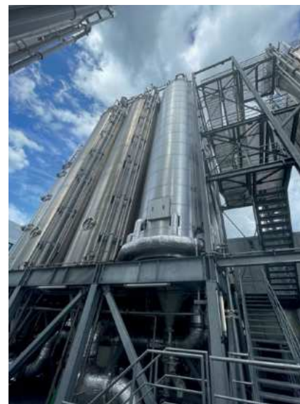
Coperion's EcoFresh silo degassing system and its twin screw extruders have received a Letter of No Objection (LNO) from the FDA and are therefore suitable for the production of food-grade HDPE and PP recyclates (Photo: Coperion, Stuttgart Germany)
